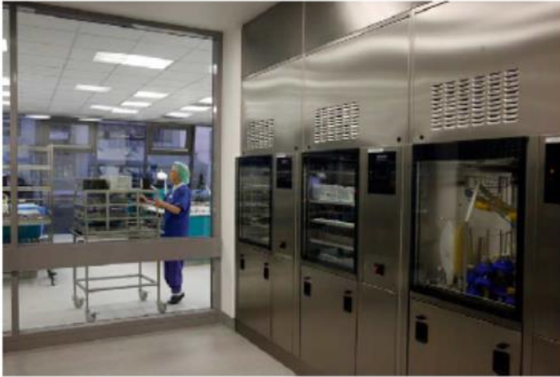
Picture 1. Example of a modern reprocessing unit for multiple-use devices. View from dirty to clean section.
